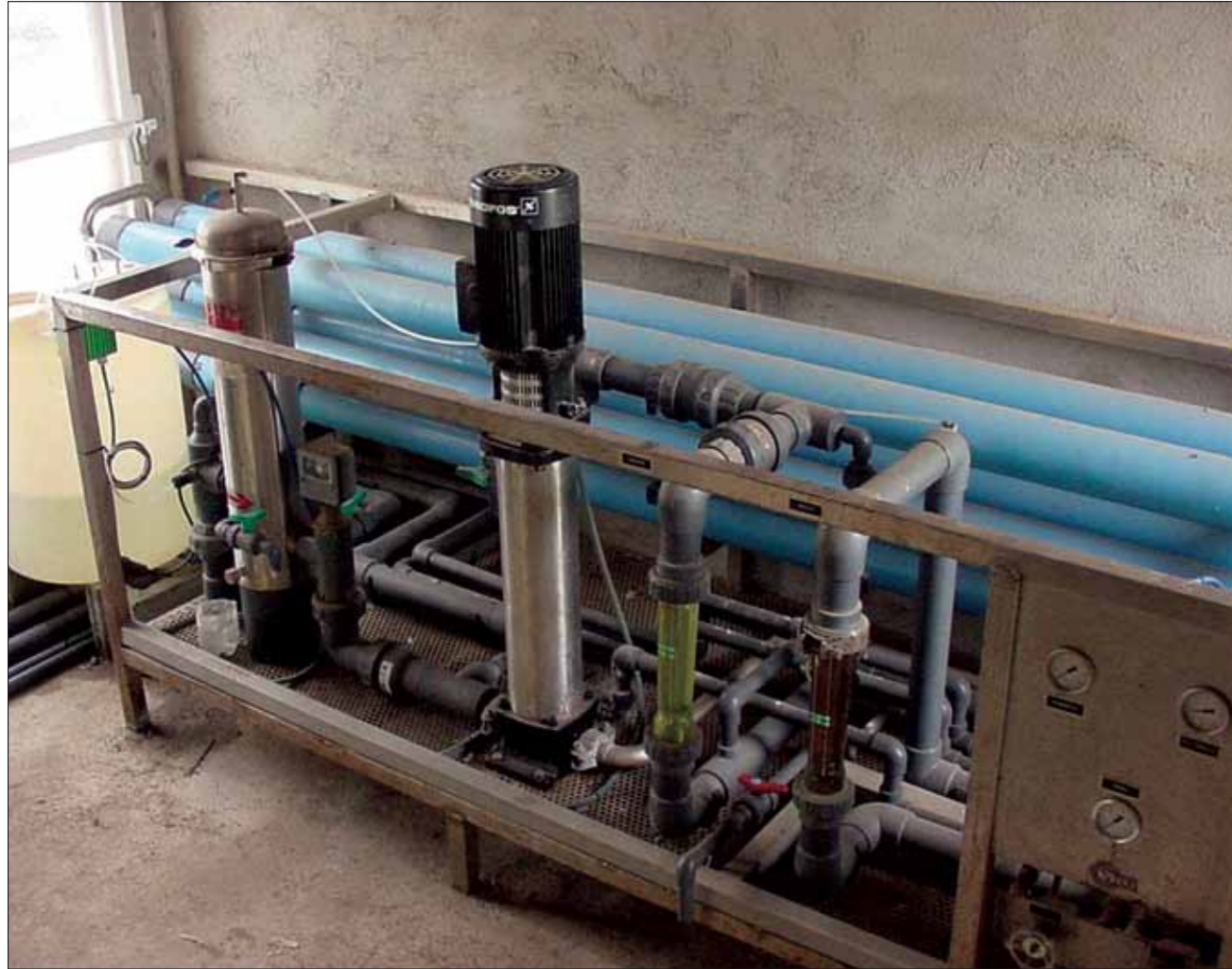
12 Reverse osmosis filtration unit used for treating water before irrigation
